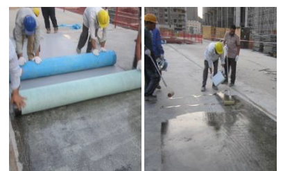
Right: Applying Proofex OFB Adhesive Left: Unrolling Proofex OFB rolls on tacky substrate
